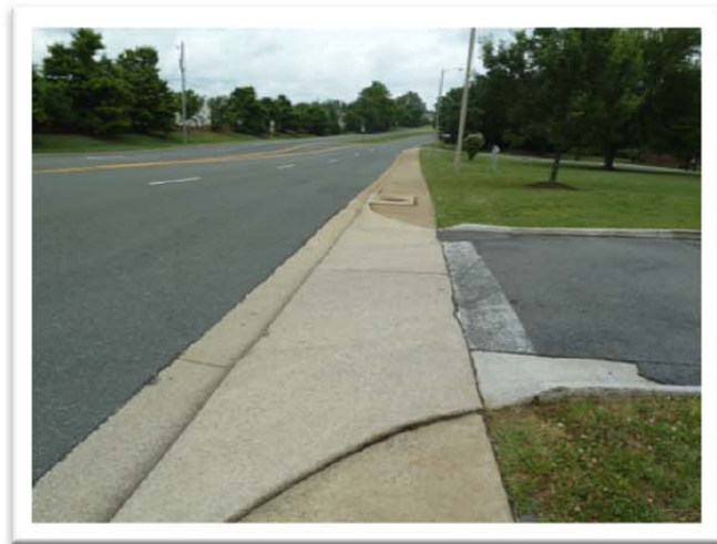
Sidewalks are only present on Mill Road in front of the school" (looking north)
