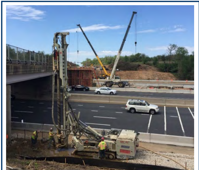
Micropiles will be used at all bridge piers so that the new foundations can be installed within the constrained site without requiring the long-term lane closures on adjacent roadways. DBT member Wagman safely installed micropiles on VDOT’s $42M Route 7 DB Project without any long-term lane closures on the Dulles Toll Road or Dulles International Highway.
